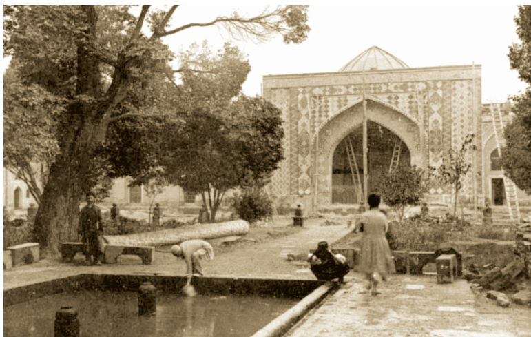
Restoration works in the courtyard of the Blue Mosque. Photo by Friedrich Sarre.
